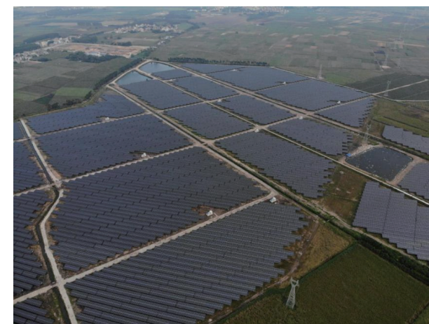
Agricultural PV Project in Yanggan Town, in Suixi County
